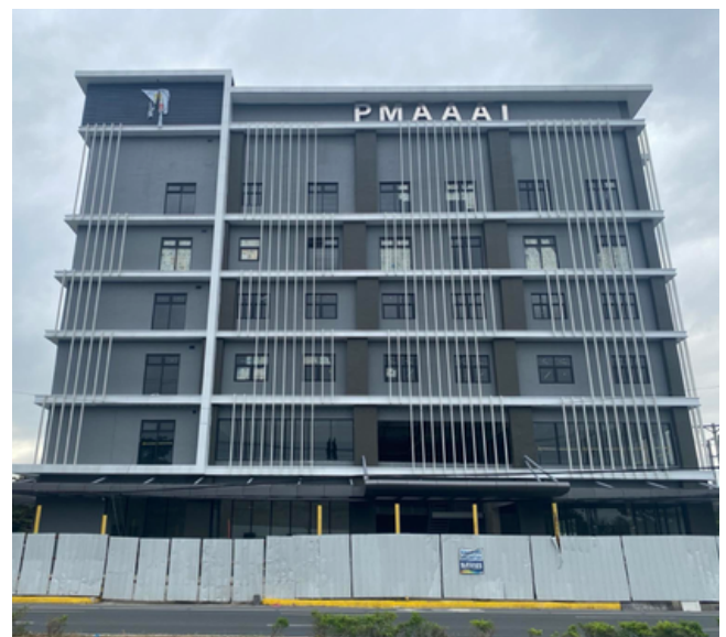
Current status of the PMAAAI Building, showing ongoing work and preparations toward project completion.
